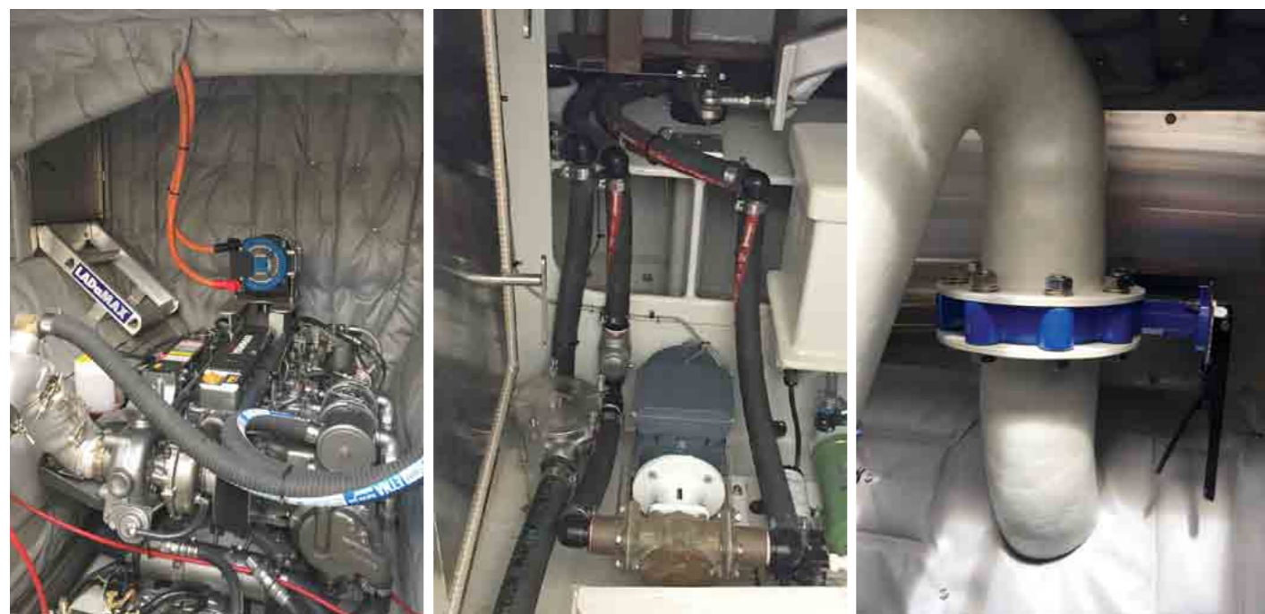
ABOVE LEFT: Engineroom with rough water access, custom fire cladding and military spec alternator mounted on custom frame bolted to engine.
